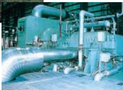
Ethylene center compressor station
